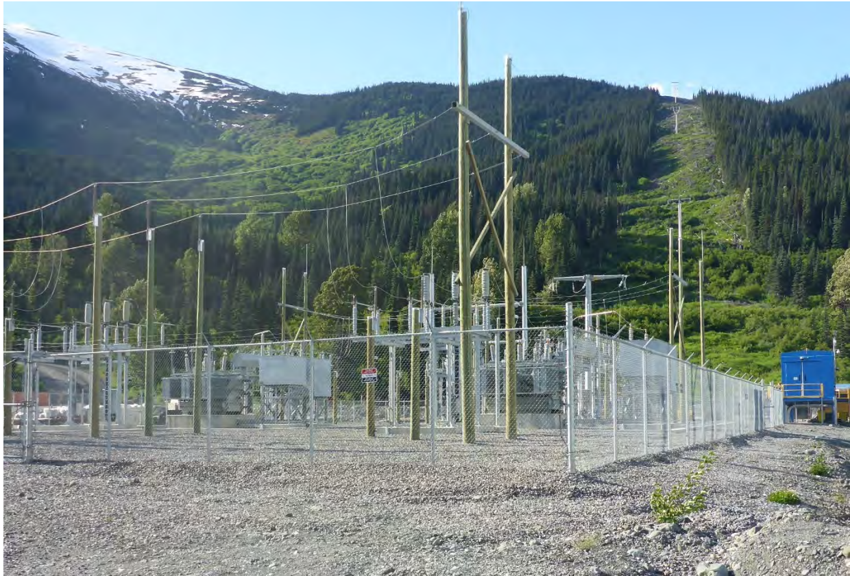
Figure 3.3-8. Knipple Substation, July 2020.
