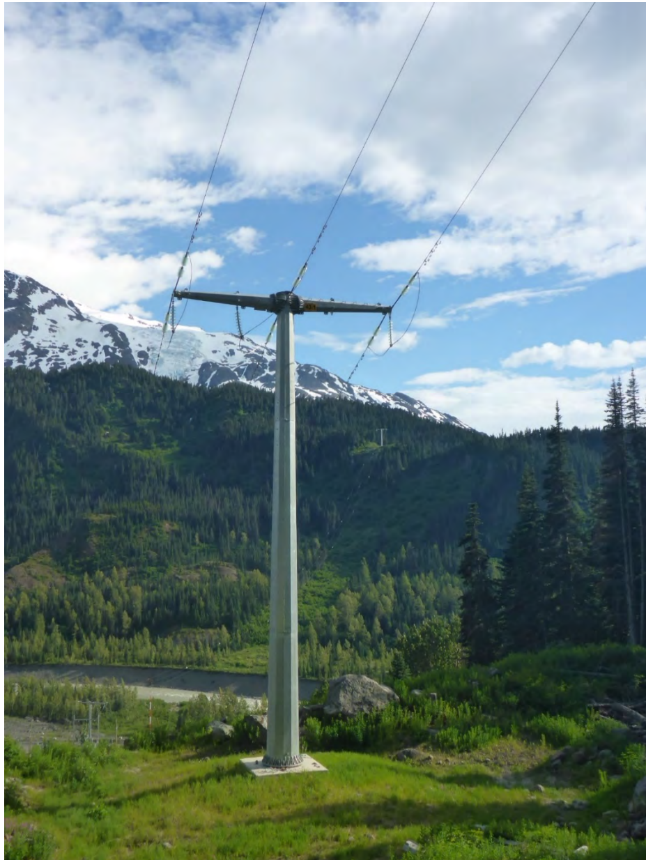
Figure 3.3-9. Seeded Transmission Line Tower Site (Photo July 2020).
