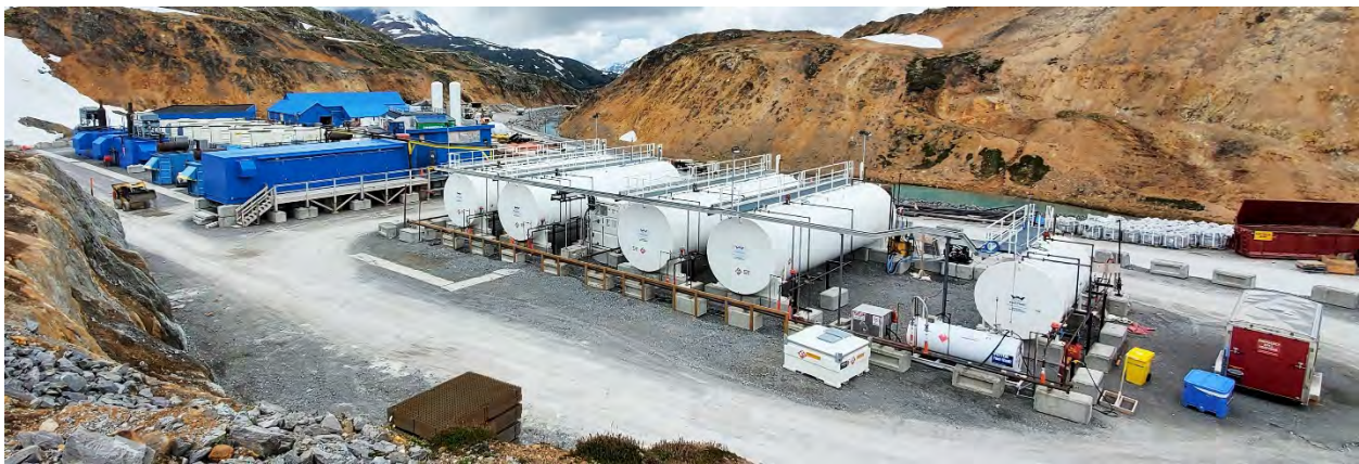
Figure 3.7-15. DPS Pad Facilities (Photo July 2020).
