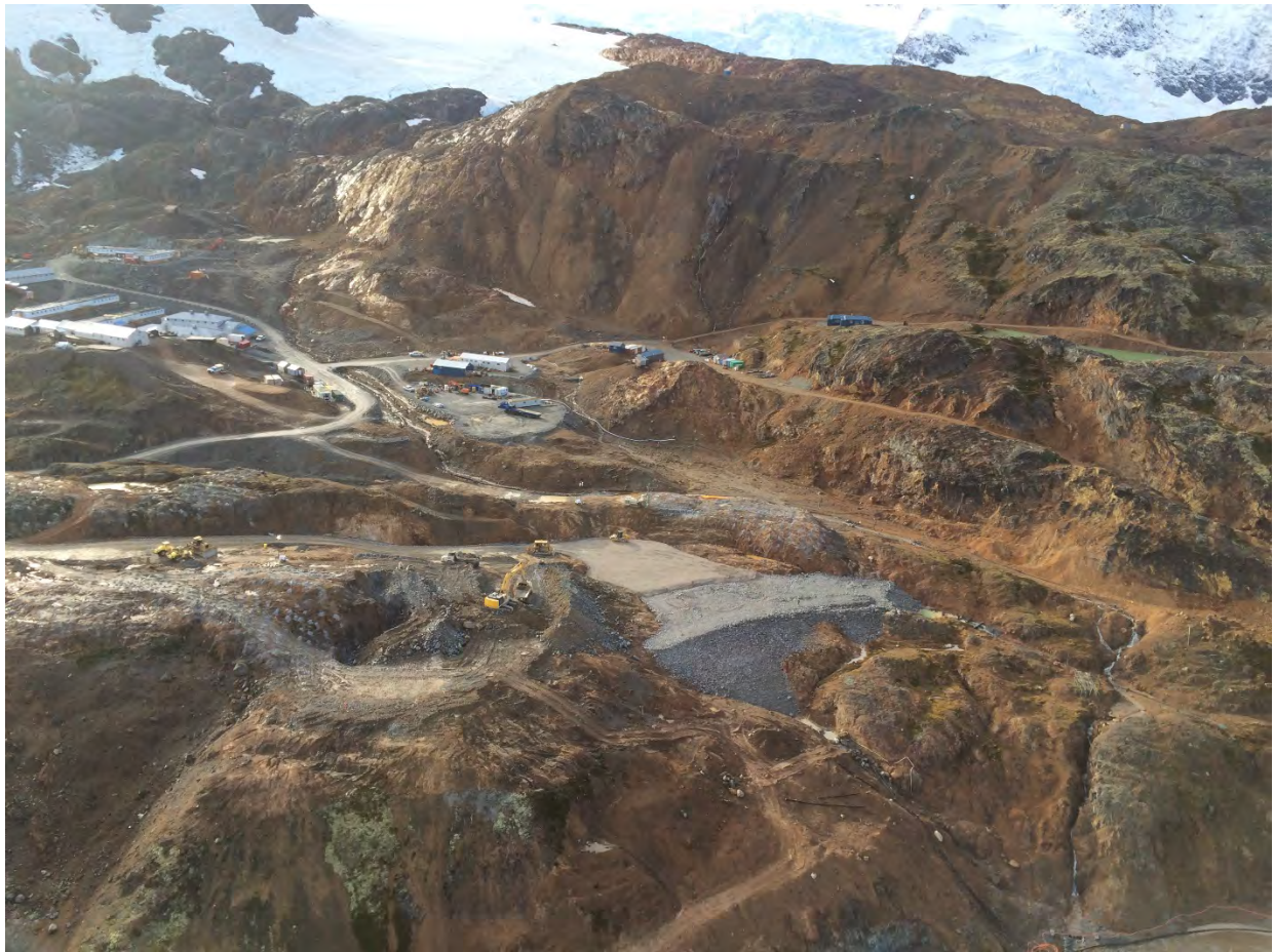
Figure 3.3-6. Development of Mine Site Level Pads During Construction with PAG Bedrock Excavation and Quarried NPAG Rock Fill, October 2015.
