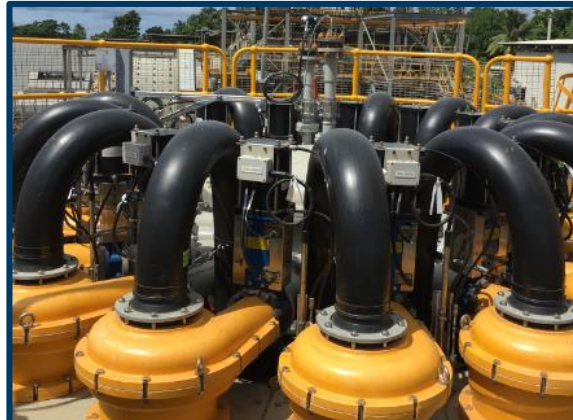
Float residue scavenging
