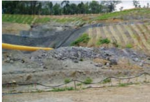
Initial decline works with ventilation at the Kencana underground mine in Indonesia.
